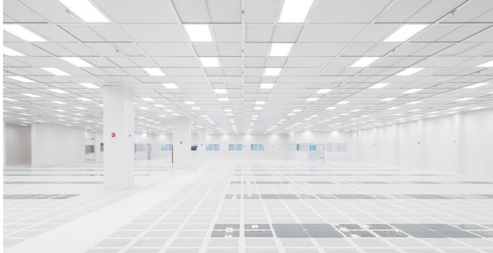
Figure 18- Open Ballroom Configuration Cleanroom with Raised Access Flooring and Recessed Elevated Waffle Slab- Note perforated RAF panels and Grated Panels for Airflow coordinated with Tool and Equipment Layouts
