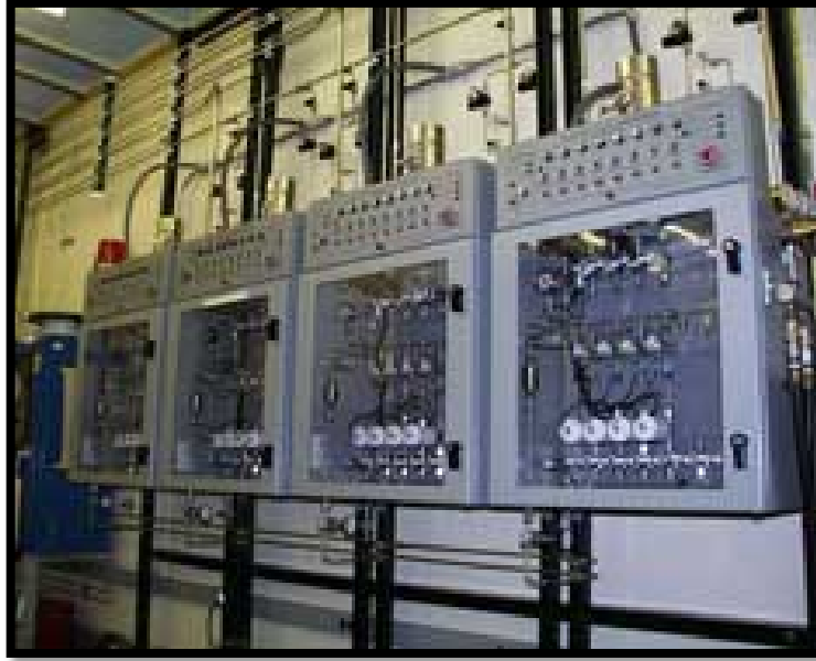
Figure 30- Valve Manifold Boxes (VMBs)
