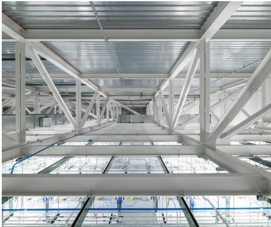
Figure 16- clean interstitial area over cleanroom/fab area with appropriately specified epoxy and intumescent coatings
