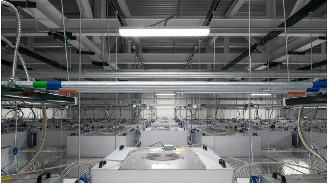
Figure 22- Walkable Clean Interstitial Space with Defined Pathways, Utility Routings, and Fan Filter Units
