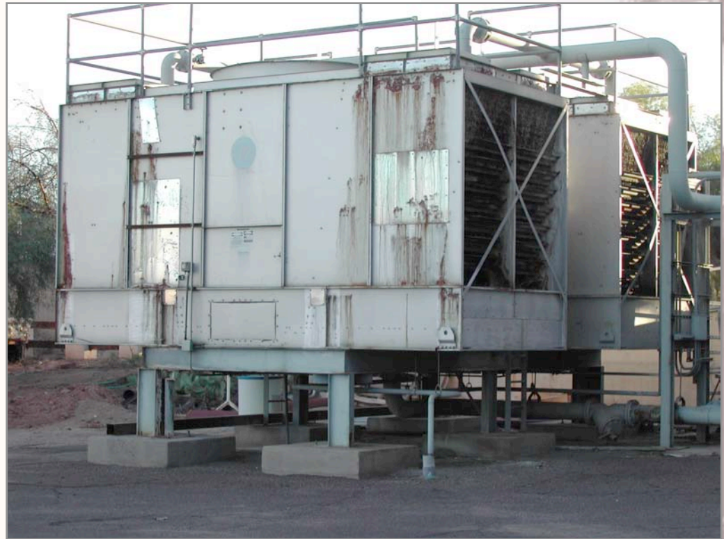
The cooling towers at the Community Services building are well beyond their useful service lives. The HVAC system is original to the building.
