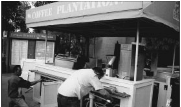
Alvino Valdes, left, and Mel Moshier of Grandville Plumbing & Piping work on one of two satellite locations of Coffee Plantation. The Coffee Plantation stands are located at the intersection of Palm Walk and Tyler Mall and next to the Business building. The stands will be open of 7 a.m. to 5 p.m. Monday through Friday, and serve coffee ranging from $1 to $3.50.
